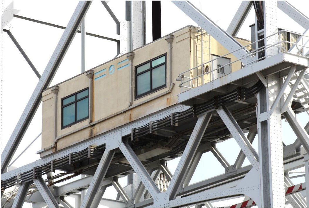
Condition Photo 1: Operator's house, including electrical conduit and access platform on west tower.
