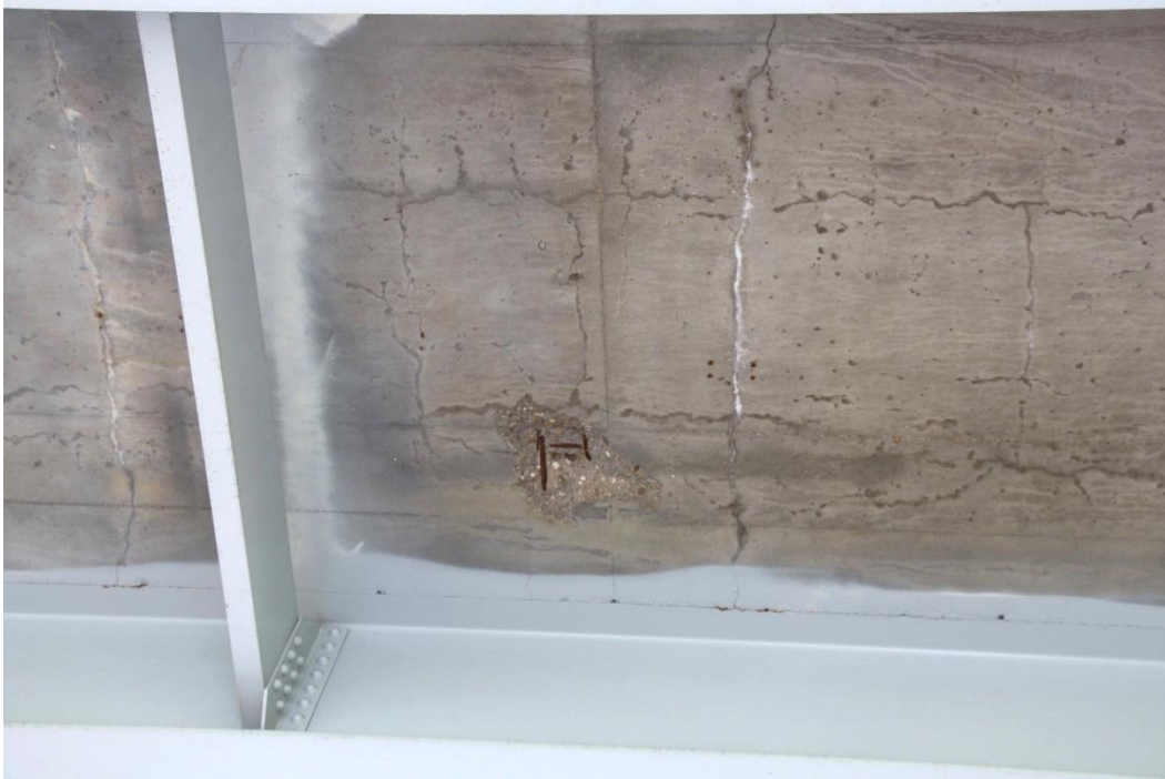
Condition Photo 23: Spalls with exposed rebar in middle of concrete deck on the underside, typical in Spans 17 to 20.
