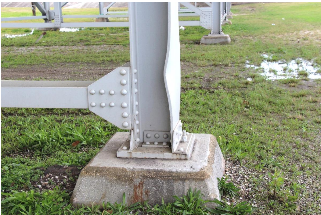
Condition Photo 20: Bent 16, north Column 1 at Jourdan Avenue has collision damage.
