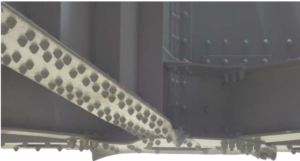
Condition Photo 22: Floorbeam 7 of the lift span left and right side has collision damage. Photo courtesy of the LADOTD.
