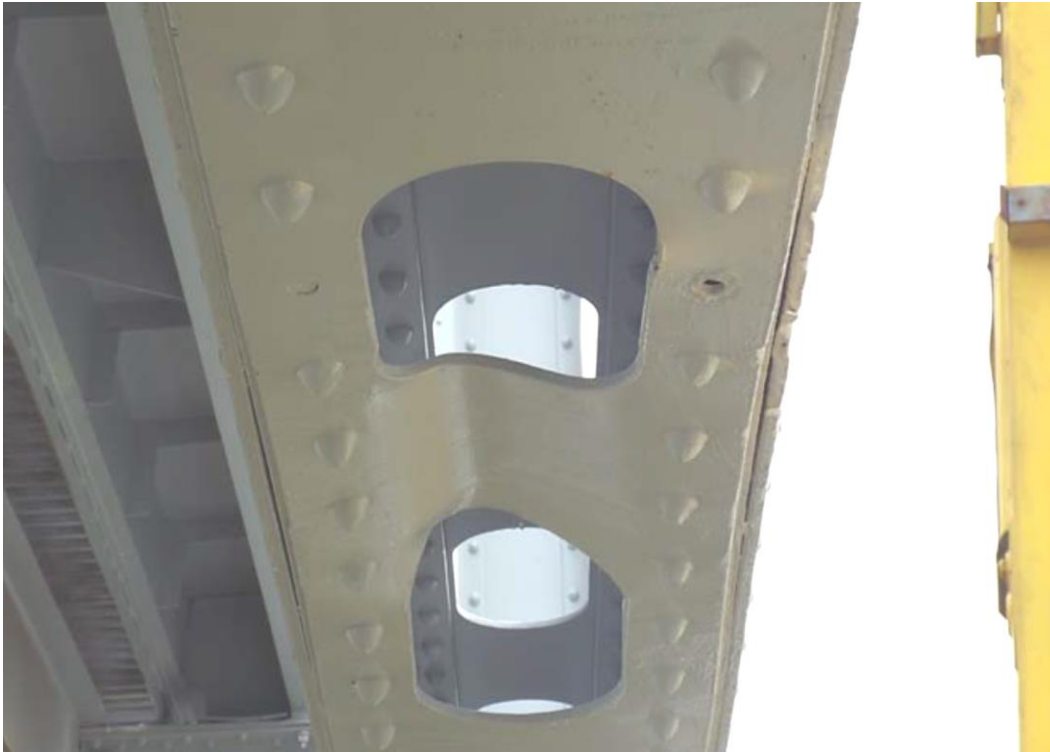
Condition Photo 21: Right side of lift span bottom chord at Floorbeam 7 has collision damage and is missing two rivets. Photo courtesy of the LADOTD.
