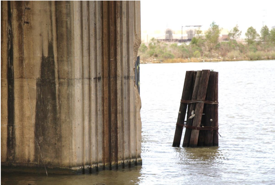
Condition Photo 19: Spalled concrete and exposed rebar at northeast corner of east tower pier.
