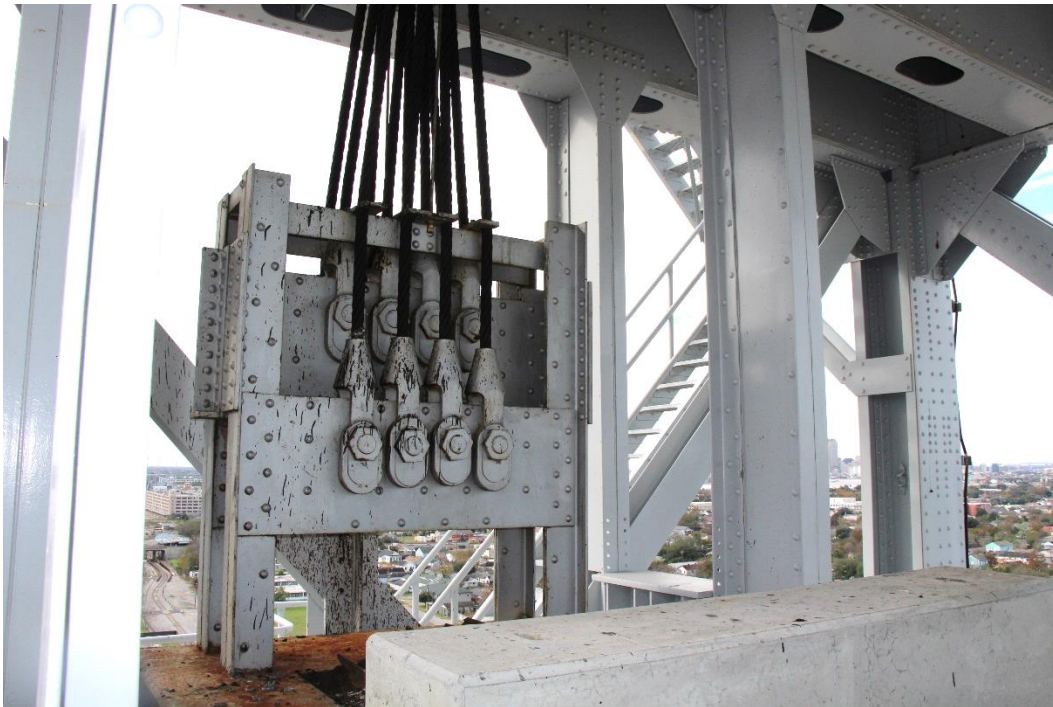
Condition Photo 8: Cables and attachment sockets to counterweight.
