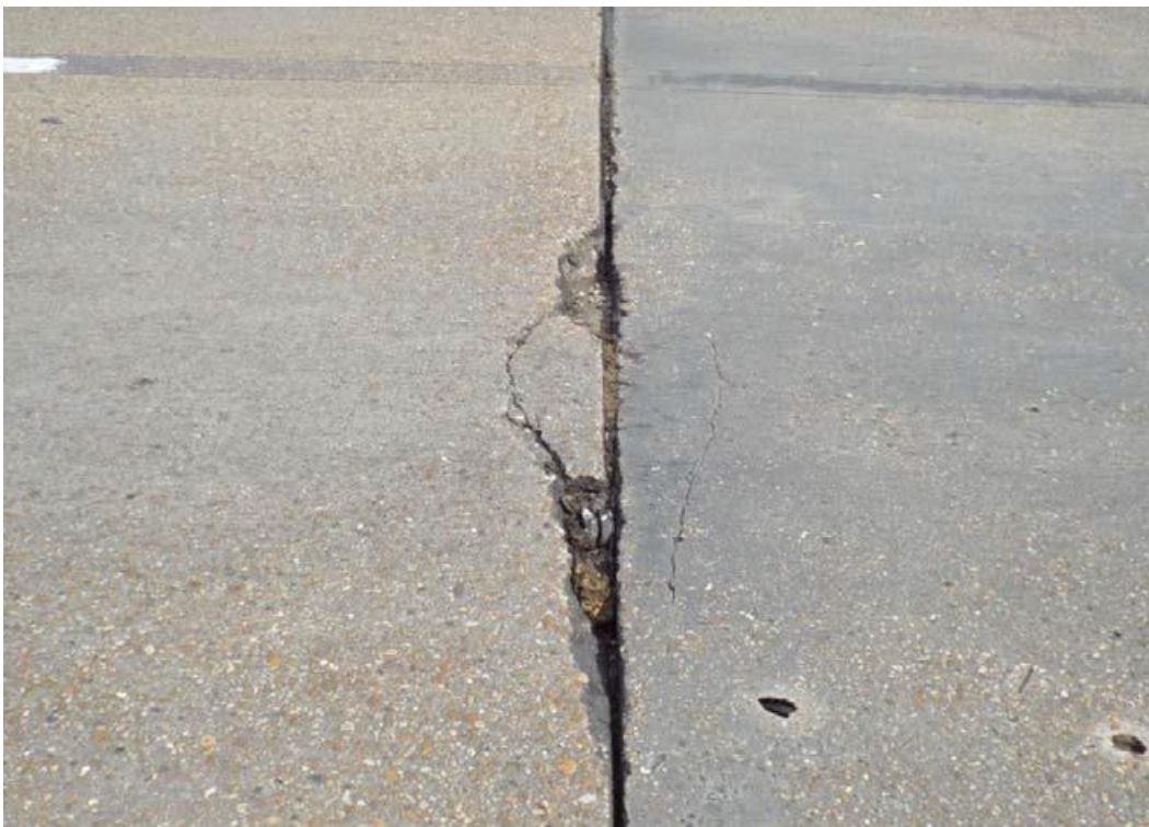
Condition Photo 24: Deck joint seals are failing and minor spalls are developing at the joints in the easterly approach spans.
