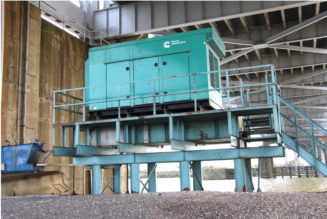
Condition Photo 3: Emergency generator under west tower.
