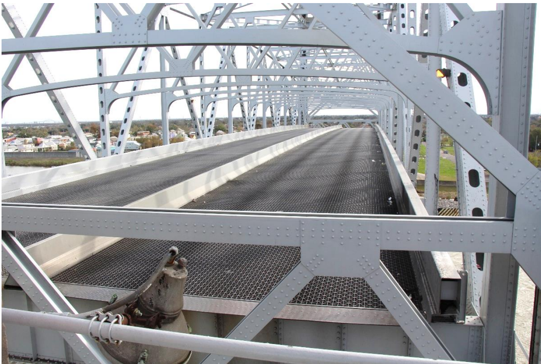
Condition Photo 4: General condition of lift span open steel grid deck, barriers, and painted steel members.
