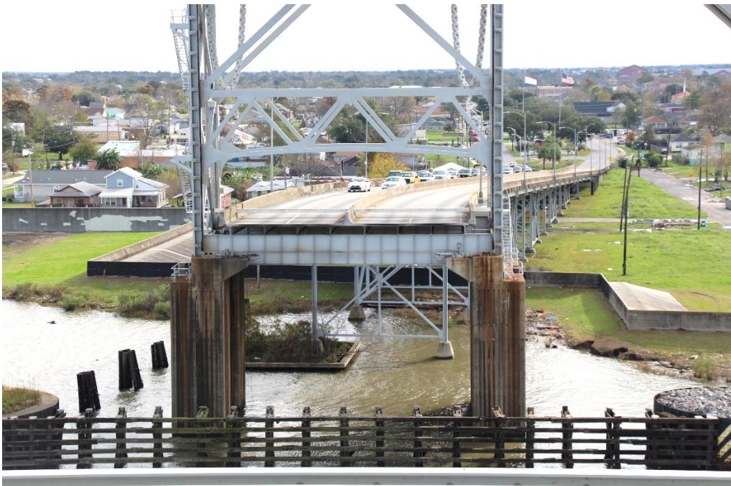
Condition Photo 6: Easterly approach spans, timber fender system, east tower, and east pier.
